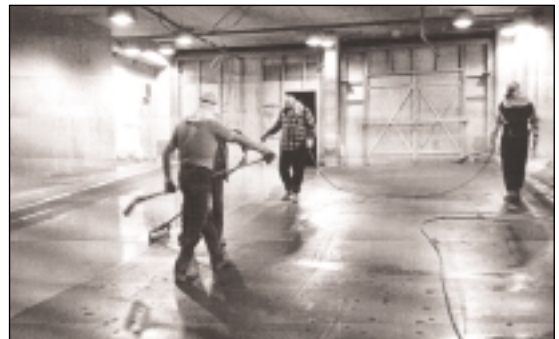
Figure 1. Application of an elastomeric waterproofing membrane system by spraying and back rolling
